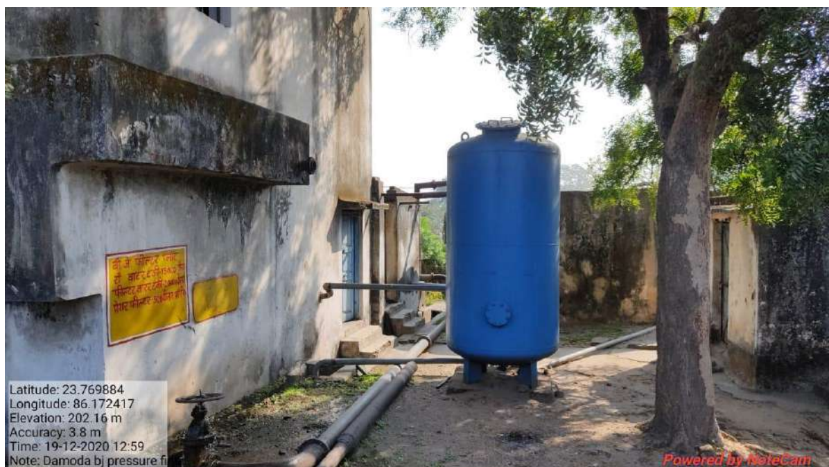
FILTER PLANT IN THE MINE AREA
